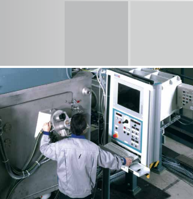
Local operation panels
